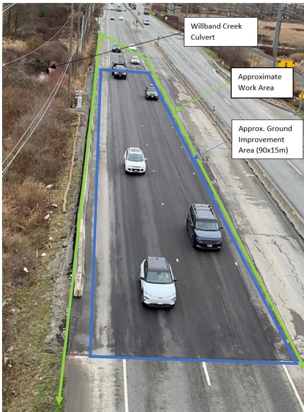
Photo 2: Southward view toward Valley Road of the moderately distressed northbound of Highway 11, January 2023.
