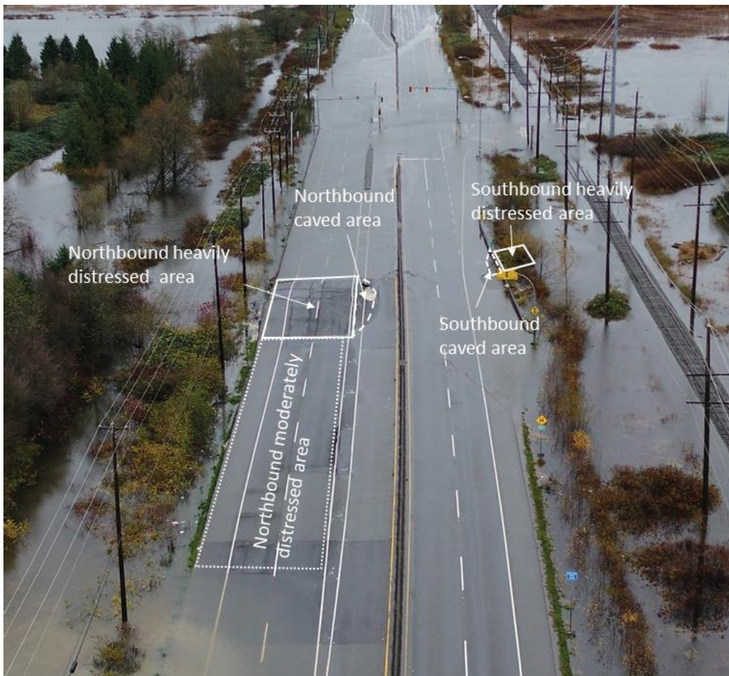
Photo 1: Southward view toward Valley Road of the distressed zones of Highway 11, March 2022 (WSP 2022a).
