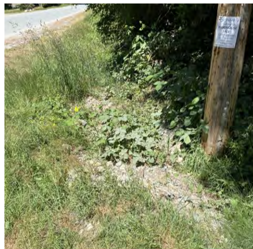
Figure 14: Beach Ave and Margaret Rd Intersection – Plugged culvert inlet
