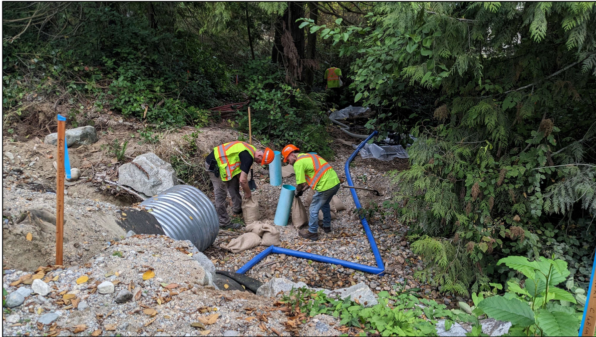
Photo 2. Works occurring in the dry channel with the dewatering hose pumping water through the culvert.
