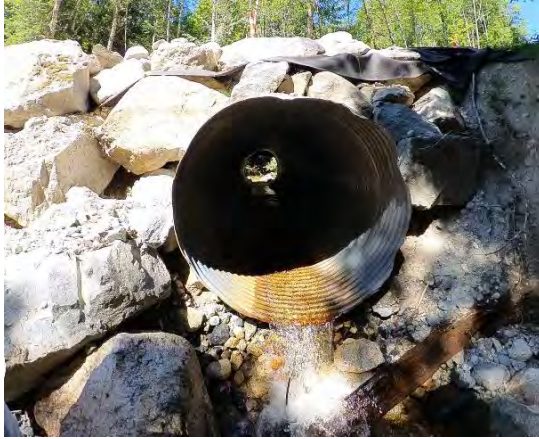
Figure 3: Day Rd – Gough Creek Outlet
