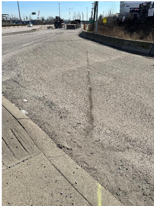
Photo 4: Moderate to High Severity Raveling at EB Turn Lane (NB Sherling Ave)
