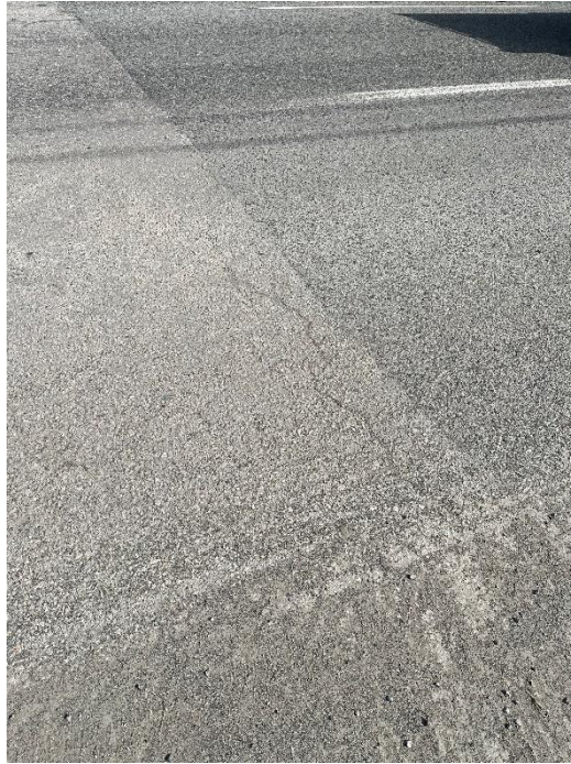
Photo 3: Low Severity Traverse Cracking Near Sta. 101+00 (Eastbound Hwy 7)
