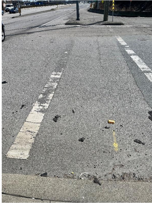
Photo 1: Moderate Severity Traverse Cracking At Sherling Avenue Crosswalk (EB Hwy &)
