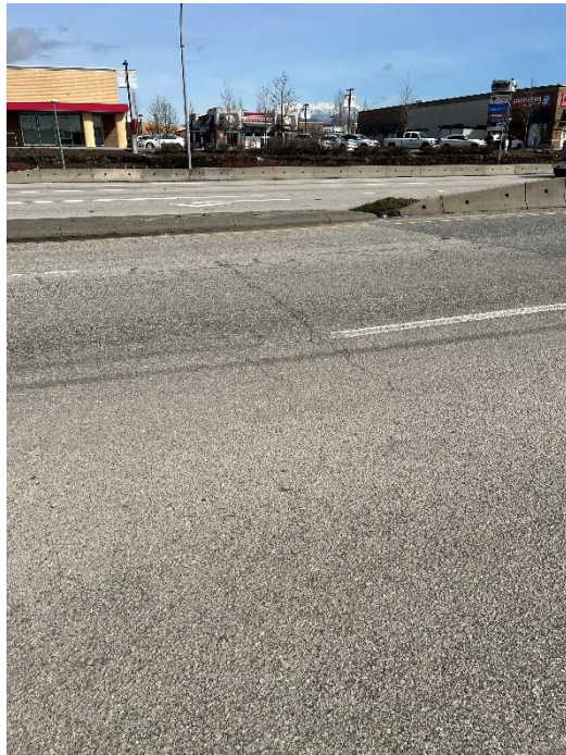
Photo 2: Moderate to Low Severity Traverse Cracking Near Sta. 100+90 (EB Hwy 7)
