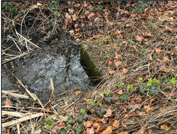
Photo 6.5 The outlet of the blocked culvert located near the existing bus stop.
