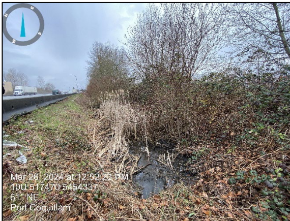
Photo 6.7 View of the start of the open-channel ditch facing east, past the existing bus stop.
