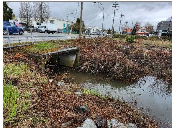
Photo 5.2 Broadway Creek culvert connecting the WB Broadway site ditch to a fish-bearing watercourse.
