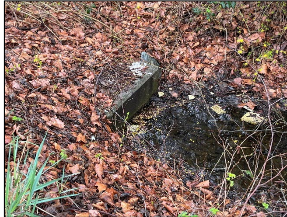
Photo 6.6 The inlet of the blocked culvert near the existing bus stop.
