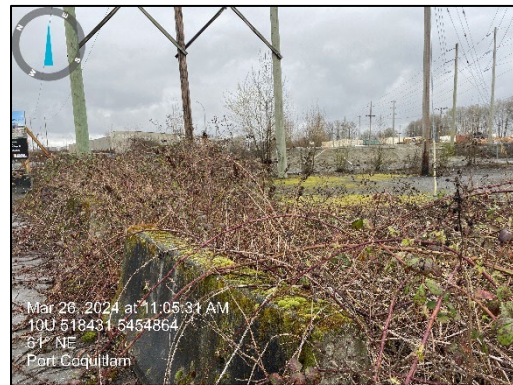
Photo 3.4 Vegetation growing along the pathway at the EB Kingsway Ave site.
