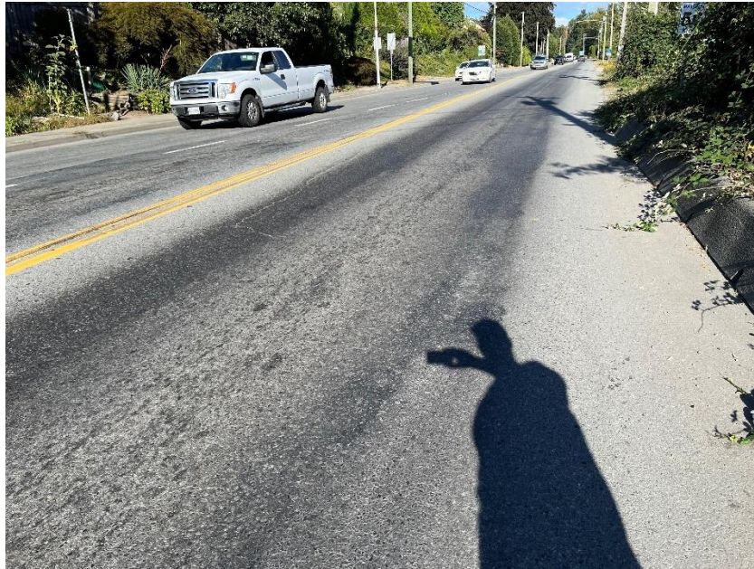
Photo 3: Moderate Severity Bleeding Near Sta. 101+50 (Eastbound)
