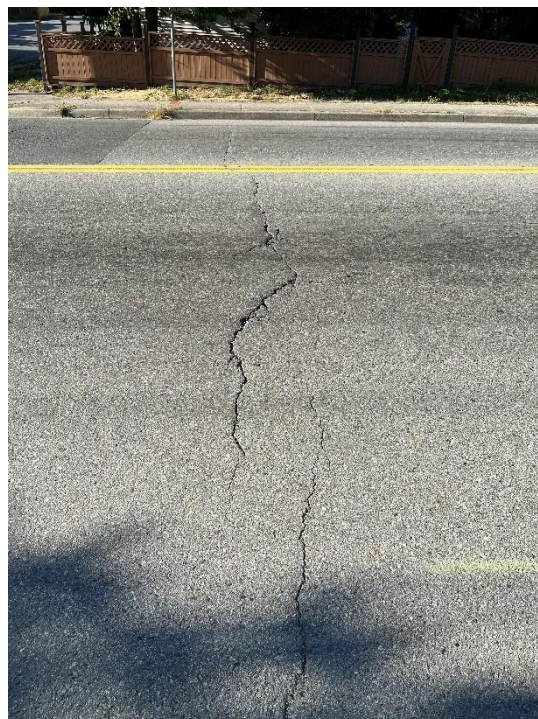
Photo 4: Moderate to High Severity Transverse Cracking Near Sta. 103+70 (Eastbound)
