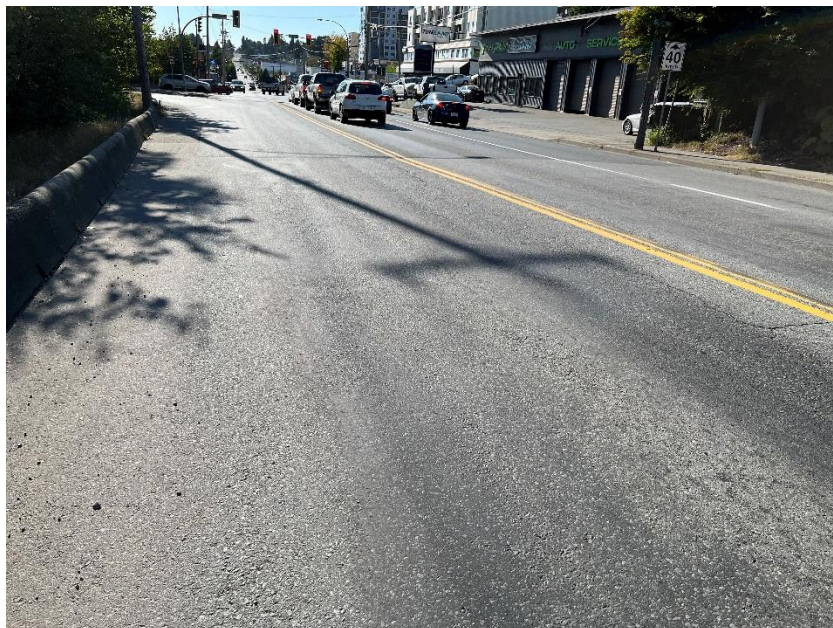
Photo 2: Moderate Severity Rutting Near Sta. 101+50 (Eastbound)
