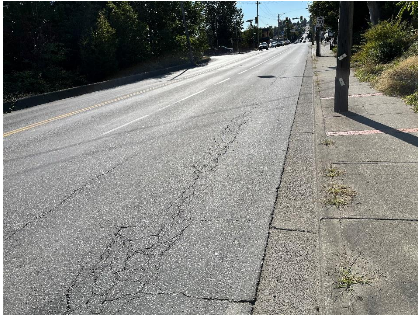
Photo 1: High Severity Longitudinal Wheel Path Cracking Near Sta. 101+50 (Westbound)
