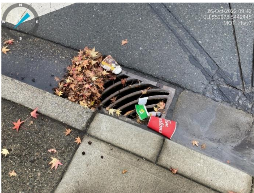
Photo 14: Open storm drain at the southern site on the eastern corner of the intersection.
