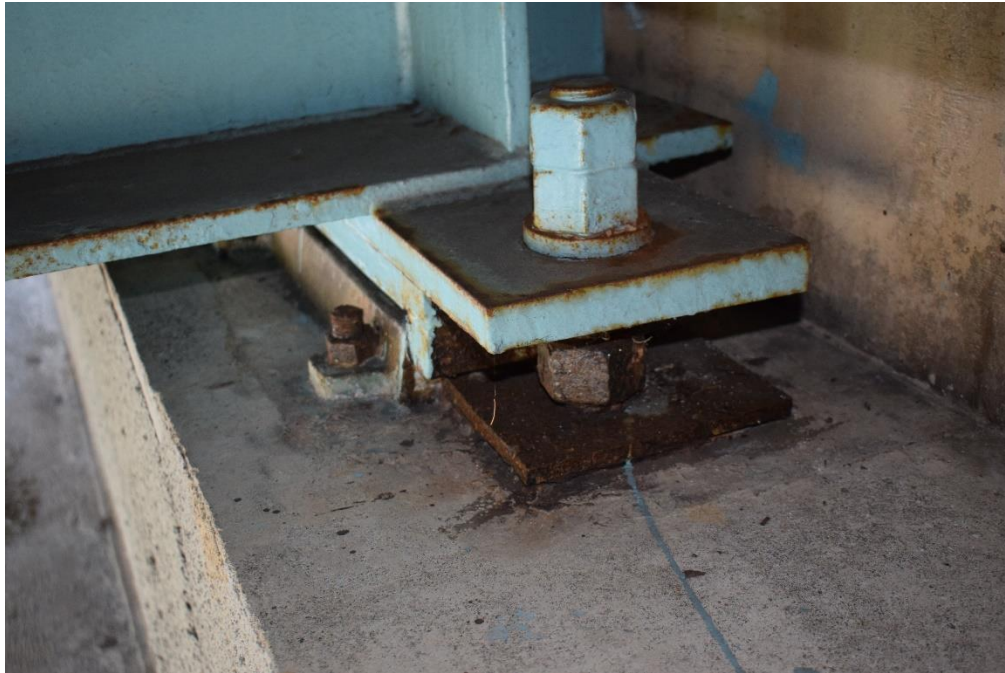
Exhibit 3.2-8: Bearing S3, Corroded Keeper Plate
