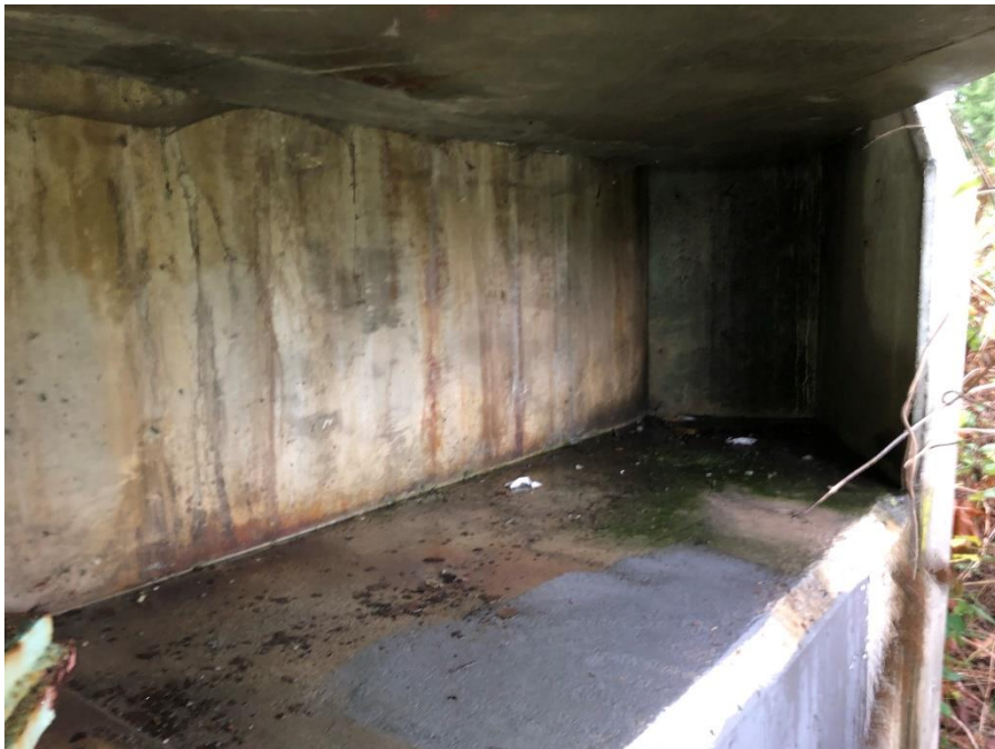
Exhibit 3.1-11: Water on South End of East Abutment Bearing Shelf
