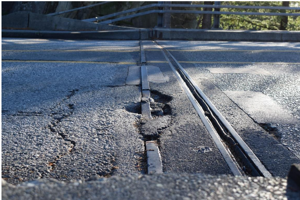
Exhibit 3.3-17: Asphalt Damage and Fractured Armoring near North Joint
