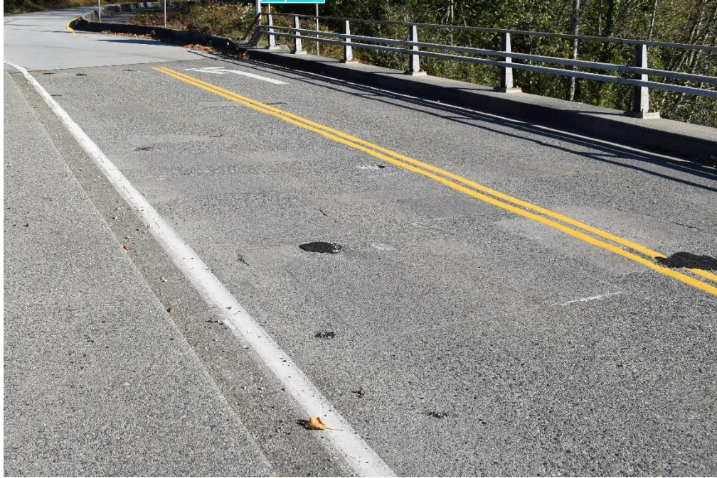
Exhibit 3.4-13: North End of Deck Surface with Repairs Visible
