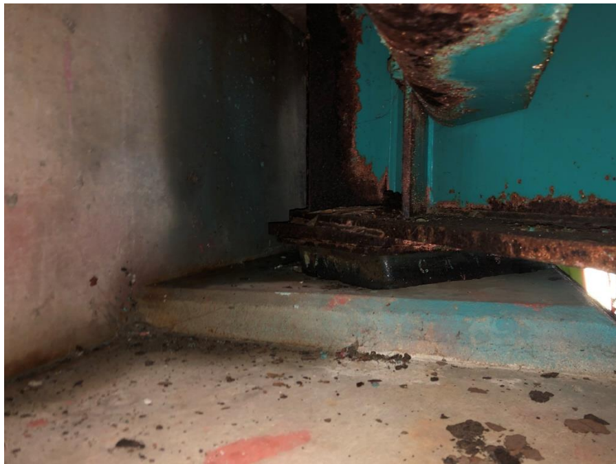
Exhibit 3.1-7: Abutment Bearing E7, Moderate Corrosion of Base Plate and Sole Plate. Typical East Abutment Bearing Condition.
