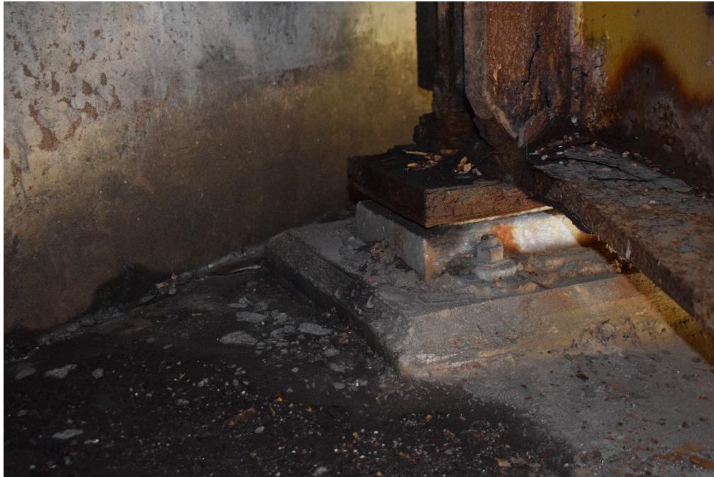
Exhibit 3.4-2: Abutment Bearing N4, Corrosion of Bearing and Girder Flange
