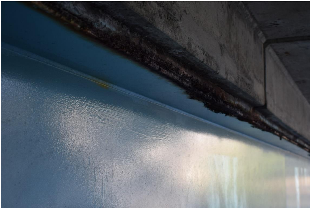
Exhibit 3.3-11: Girder 6 Top Flange Corrosion, Looking North
