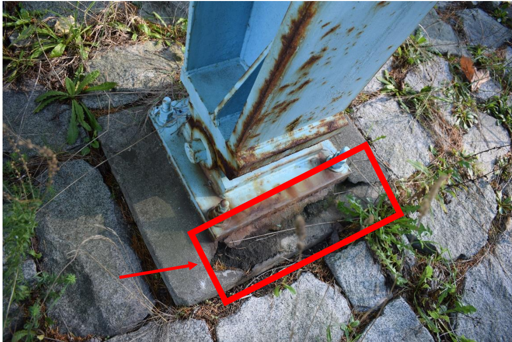
Exhibit 3.3-3: Inclined Pier Bearing N5, Debonded Grout Pad
