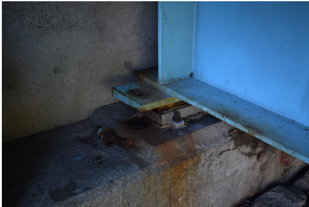
Exhibit 3.3-5: Abutment Bearing S6, Anchor Bolt Failure
