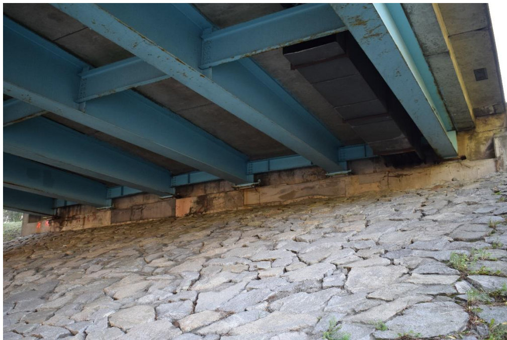
Exhibit 3.3-10: South Bearing Shelf, Cracking, Delaminations and Past Repairs Visible
