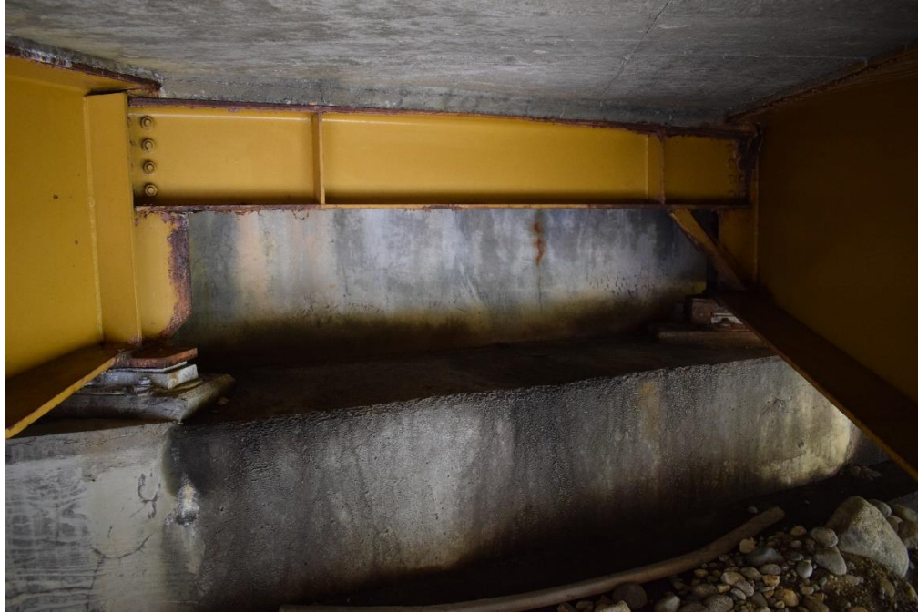
Exhibit 3.4-6: Water Stain Between Abutment Bearings N2 and N3
