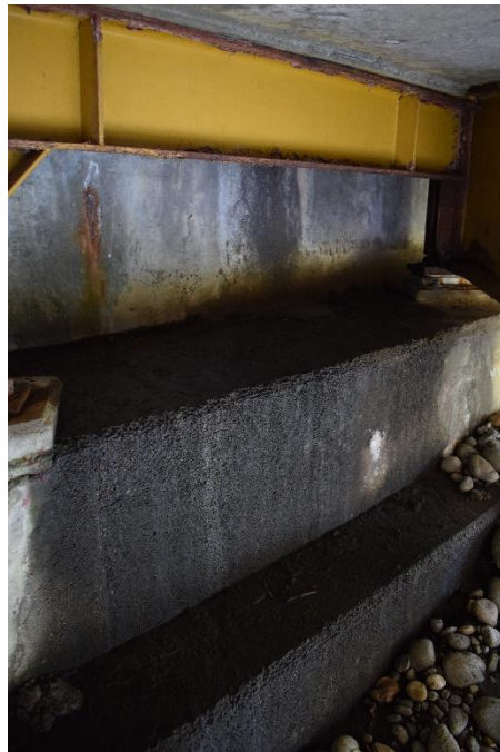
Exhibit 3.4-7: Water Stain Between Abutment Bearings N3 and N4
