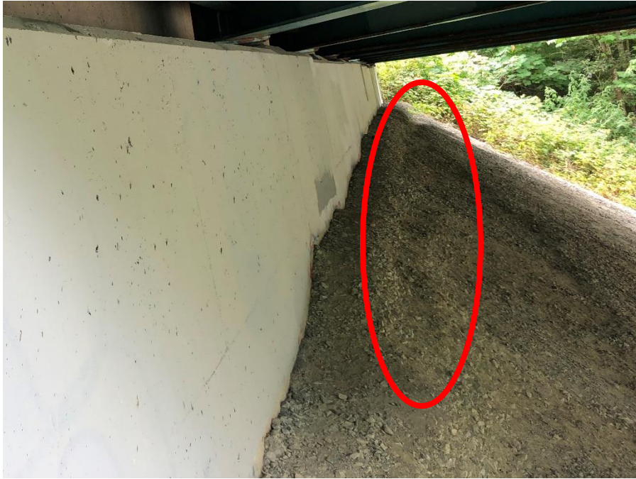
Exhibit 3.1-10: Erosion of East Abutment Slope.
