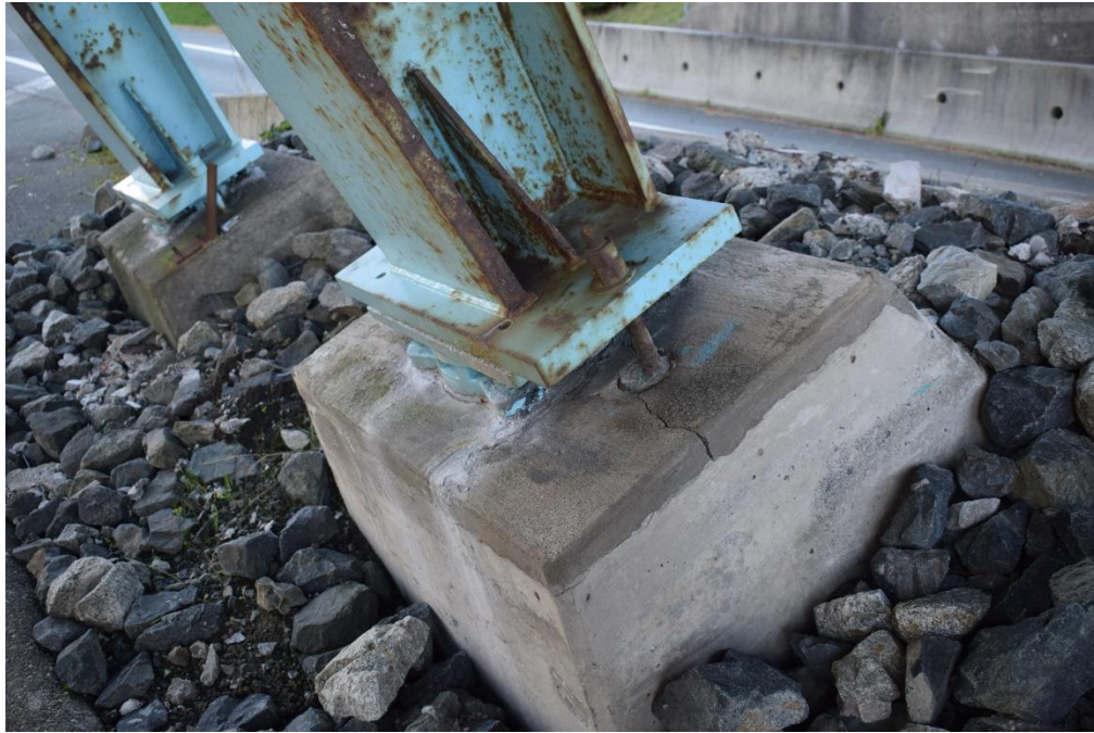
Exhibit 3.2-1: Pier S4 Bearing, Minor Corrosion on Base Plate. Crack in the Debonded Layer.
