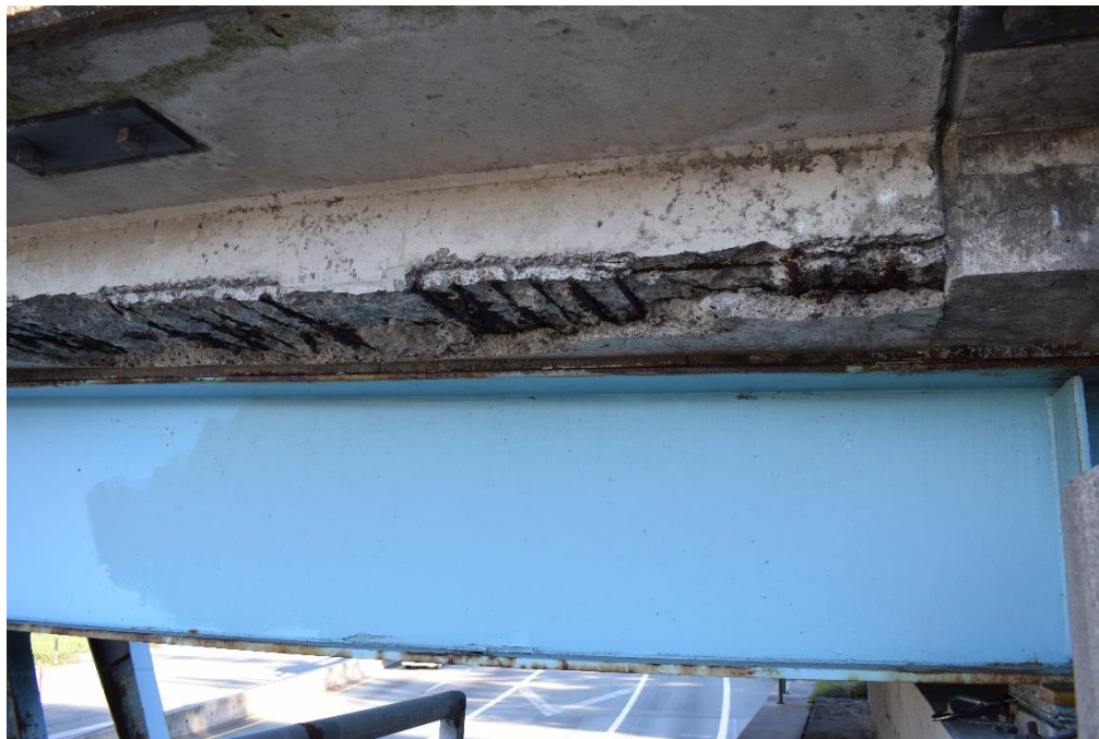
Exhibit 3.2-13: West Deck Fascia at South End of Bridge, Spalling and Exposed PT
