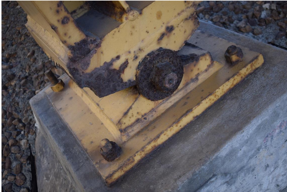
Exhibit 3.4-1: Pier N3 Bearing, Corrosion on Pin Washer and Rocker Plates
