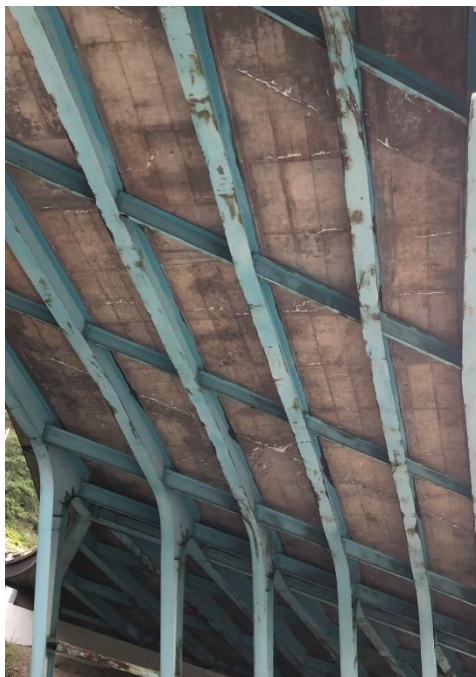
Exhibit 3.1-12: View of Steel Condition and Efflorescence on Soffit Looking East
