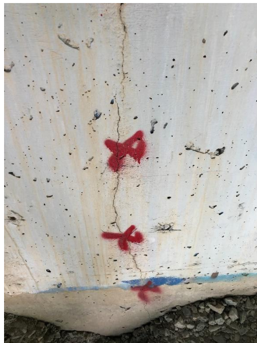
Exhibit 3.1-9: Vertical Crack Just North of Abutment Bearing E4
