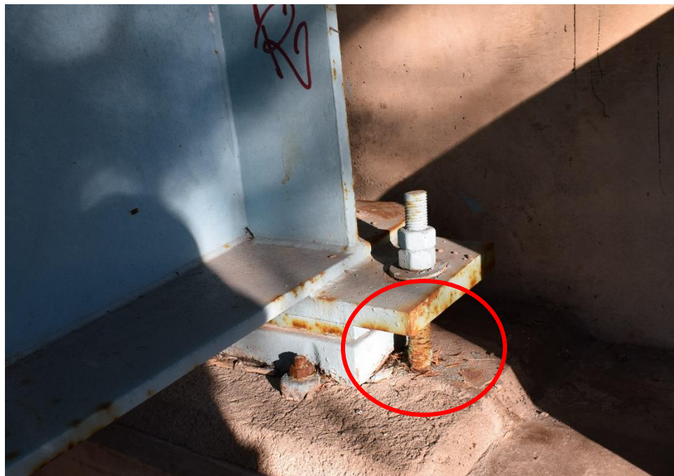
Exhibit 3.3-6: Abutment Bearing N6, Necking of Bolt Entering Bearing Shelf
