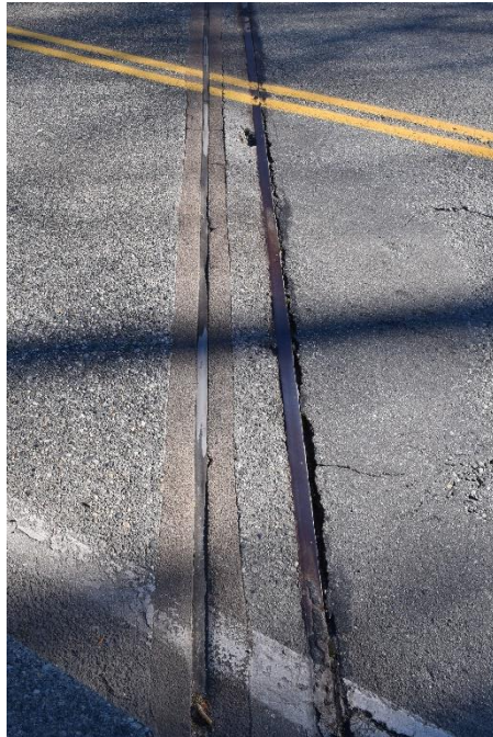
Exhibit 3.4-12: Asphalt Deterioration at South Abutment Joint
