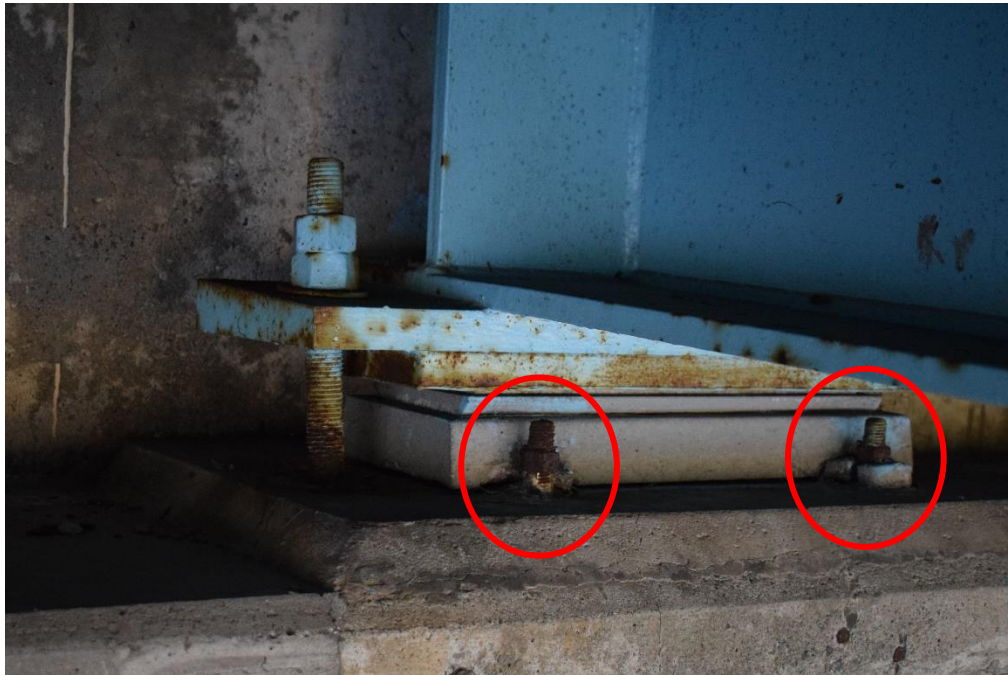
Exhibit 3.3-9: Abutment Bearing S2, Fractured Tabs on Base Plate
