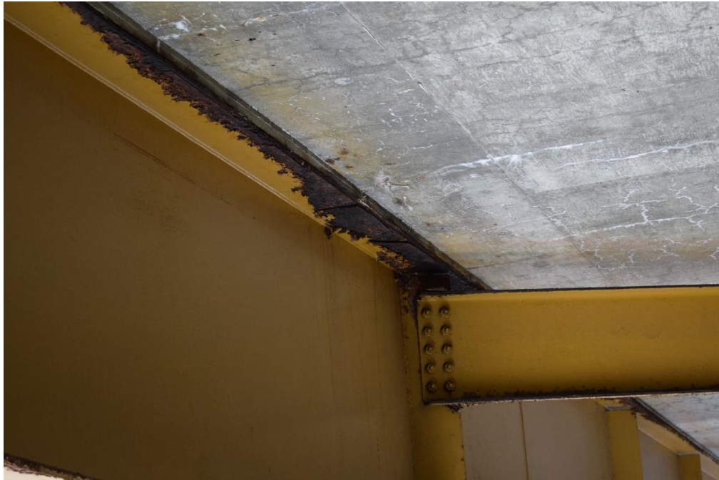
Exhibit 3.4-9: Girder 4 Top Flange from North Abutment, Localized Flaking/Section Loss
