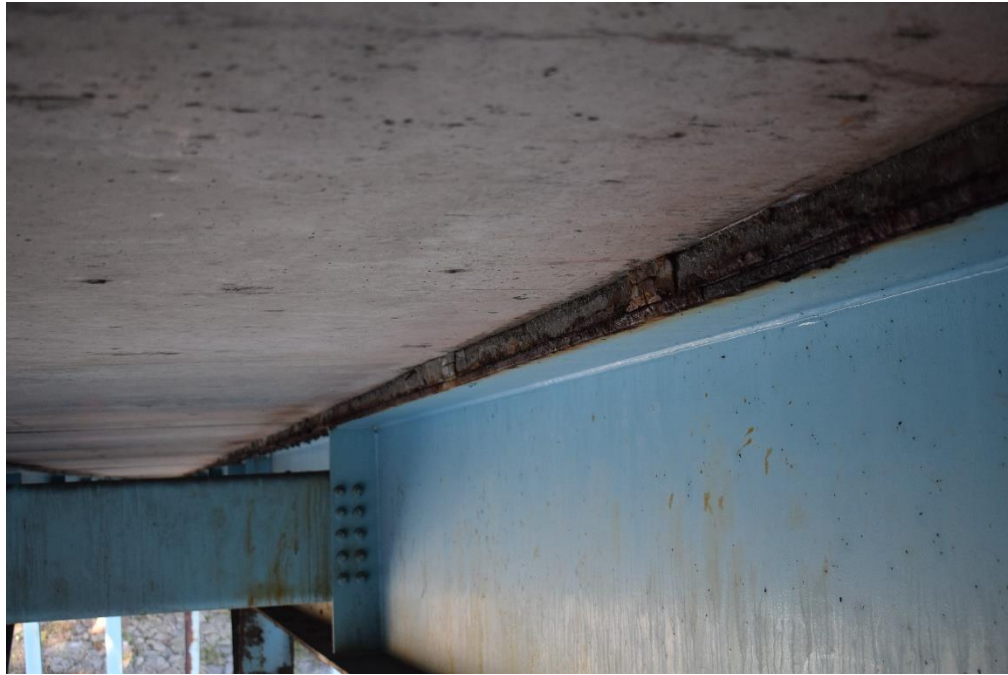
Exhibit 3.2-9: Girder 3 Looking North, Coating Loss and Corrosion Along Top Flange
