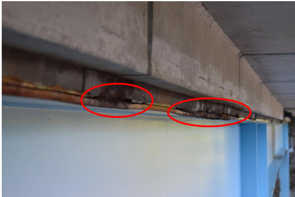
Exhibit 3.2-10: Girder 5 Looking North, Undulating Top Flange Due to Pack Rust
