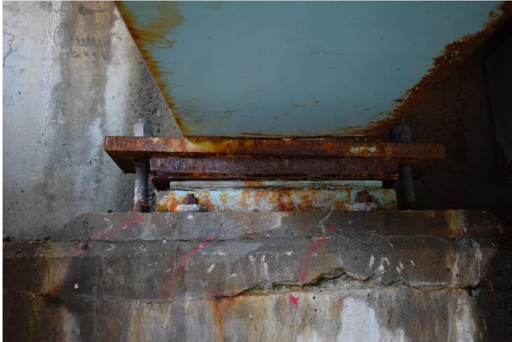
Exhibit 3.3-4: Abutment Bearing N1, Heavily Corroded
