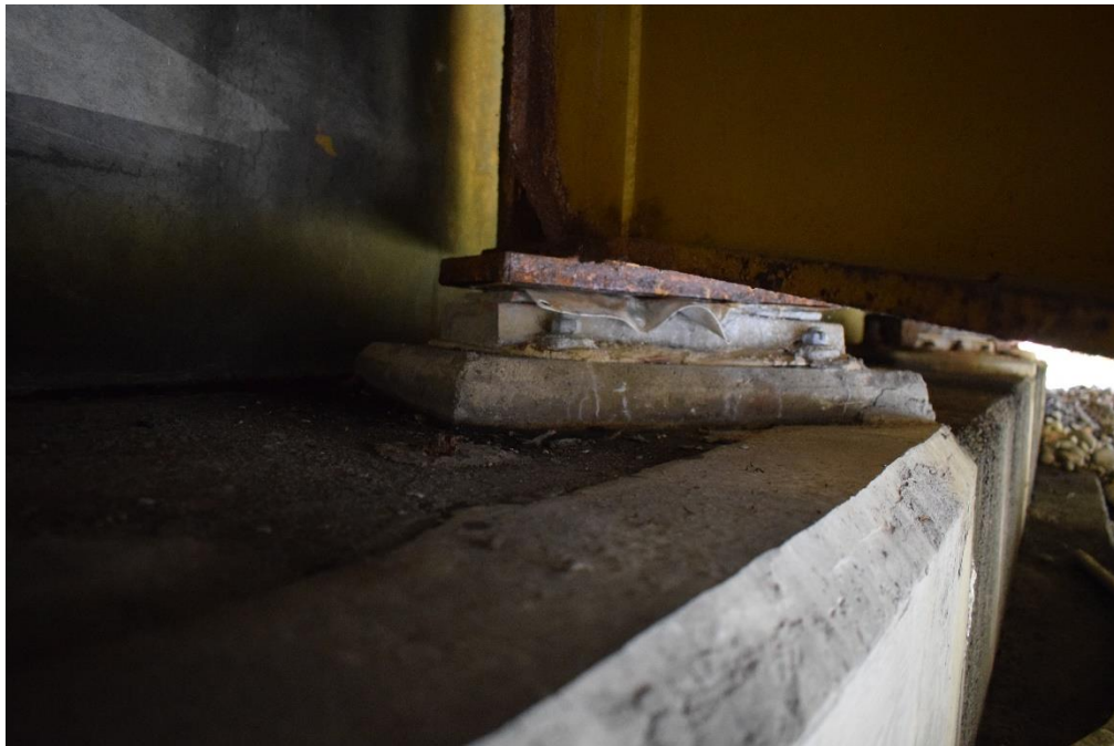
Exhibit 3.4-3: Abutment Bearing N2, Failed Polymer Sheet
