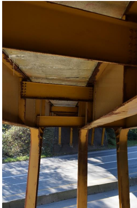
Exhibit 3.4-8: Between Girders 4 and 5 Looking South, Coating Loss Along Top Flange
