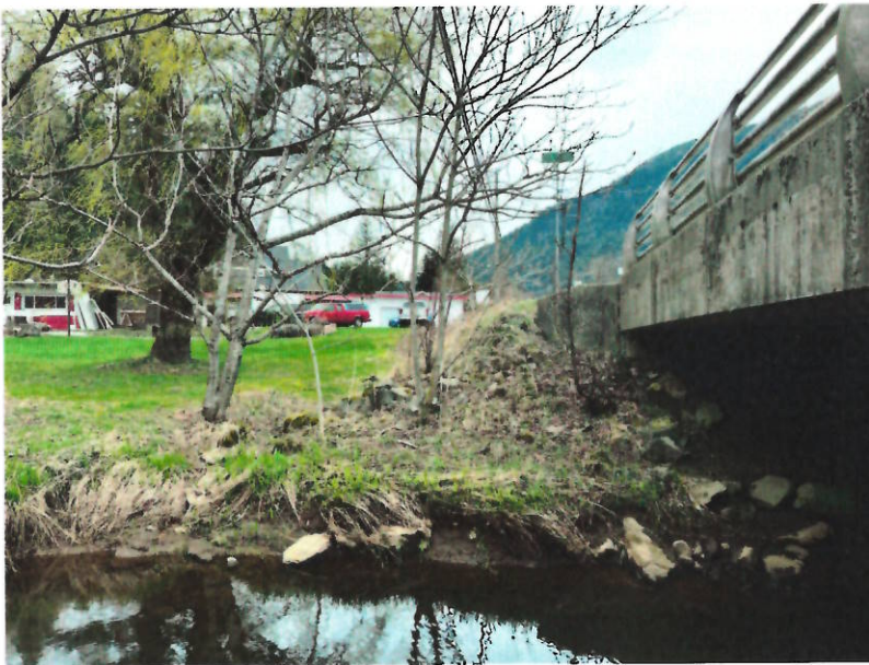
Photo 1: Looking north at the wing wall on the west side of the north abutment of the bridge. A drainage ditch with an outlet to the creek will be constructed at the toe of the embankment.
