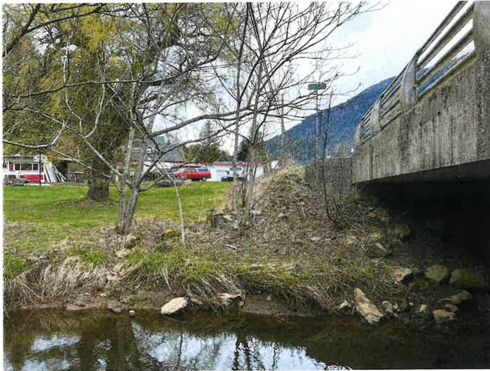
Photo 2: Looking north at the area west of the north abutment of the bridge from the south bank of the river.
