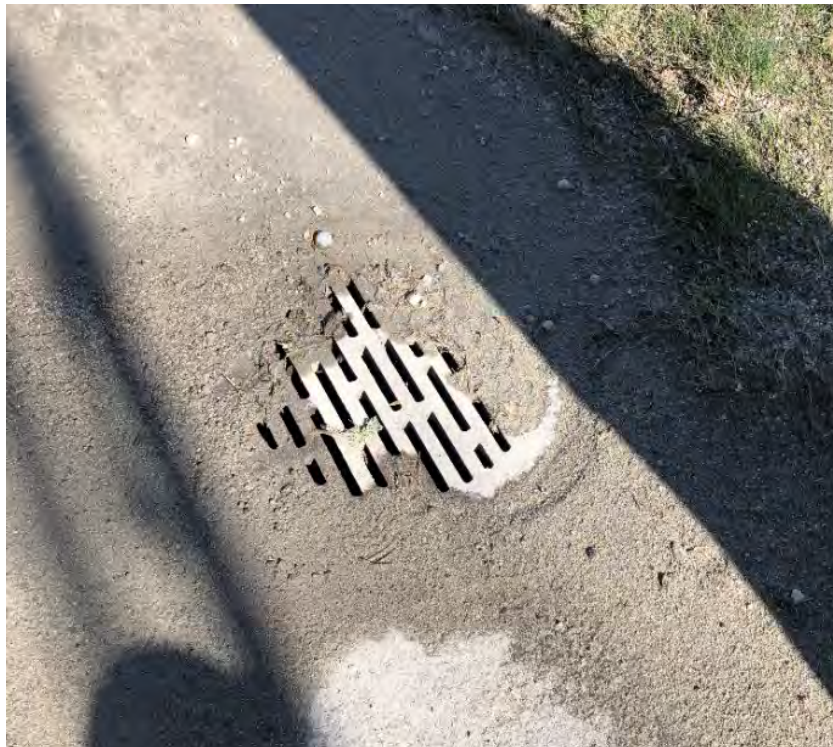
Photo 8 Catch basin located on the western shoulder of Sechelt Inlet Road, in front of Columbia Fuels at 103+40. Photo taken facing northeast.
