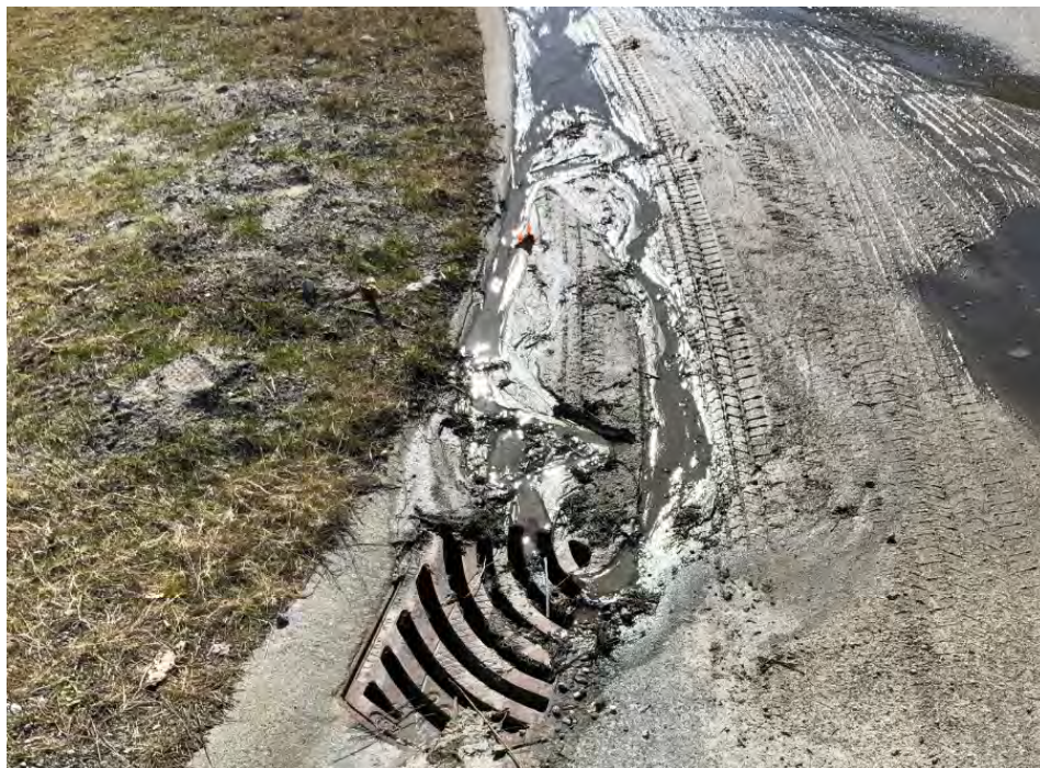
Photo 12 Catch basin located at Ikat Drive visibly receiving runoff from Sechelt Inlet Road via Tsulich Drive. Photo taken facing south.
