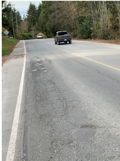
Photo 1: General Condition of the Roadway showing Fatigue Cracks
