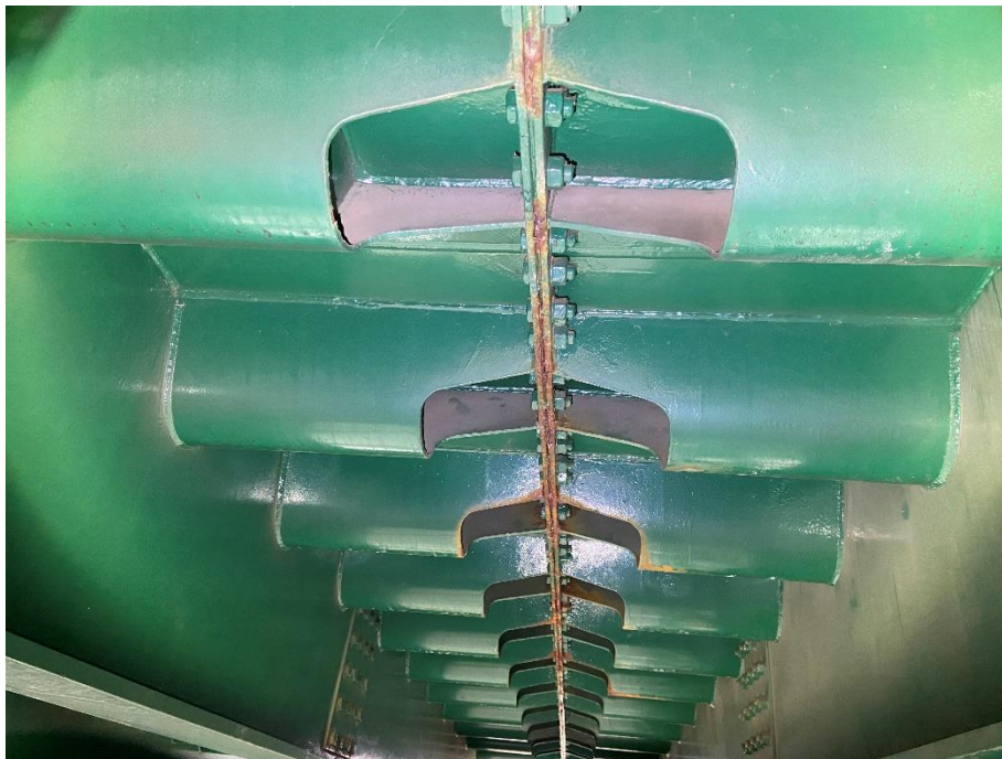
Figure 19: Splice Between Bent 4 and 5 Showing More Moisture Than Typical.
