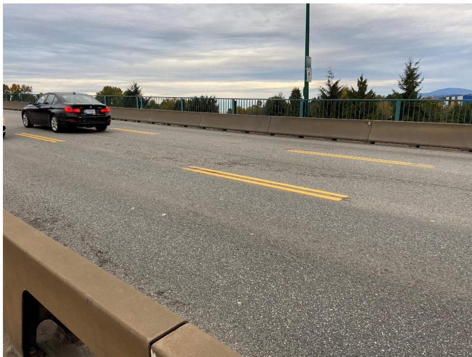
Figure 5: Typical Wearing Surface Typical Condition.
