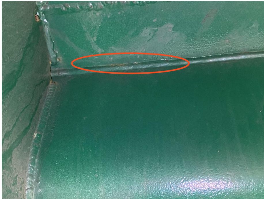
Figure 9: Minor Rusting on Longitudinal Weld on East Side of Trough 3 at 3rd Floorbeam from Bent 1 in the Direction of Bent 2.
