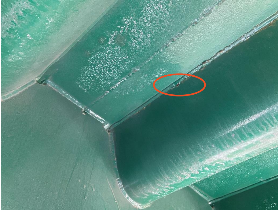
Figure 11: Localized Paint Failure on Longitudinal Weld on East Side of Trough 3 at 2nd Floorbeam from Bent 8 in the Direction of Bent 7.
