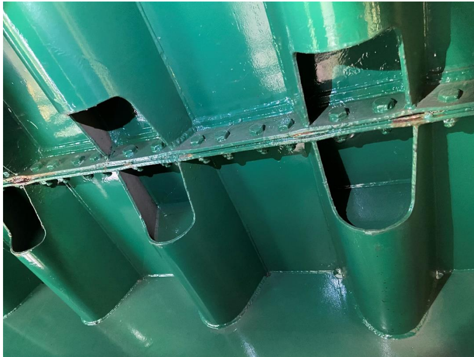
Figure 18: Rust Jacking at Splice Between Bent 19 and 20.
