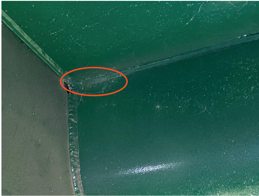
Figure 13: Minor Rusting near Termination of Longitudinal Weld on West Side of Trough 5 at 3rd Floorbeam from Bent 13 in the Direction of Bent 12.
