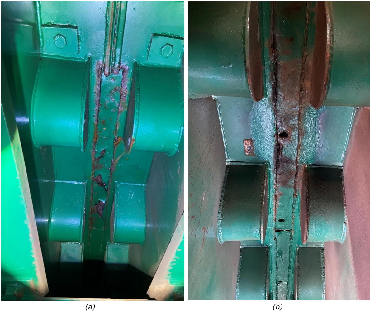
Figure 25: Poor Condition Link Plates at (a) West Side of Bent 21 and (b) Bent 3
