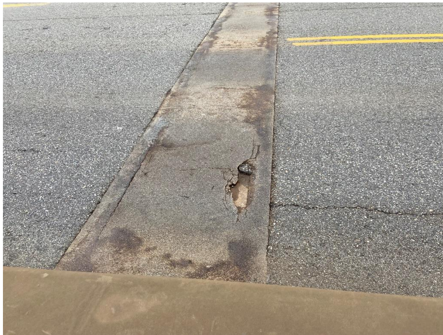
Figure 7: Localized Spalling in Wearing Surface at Link Plates.
