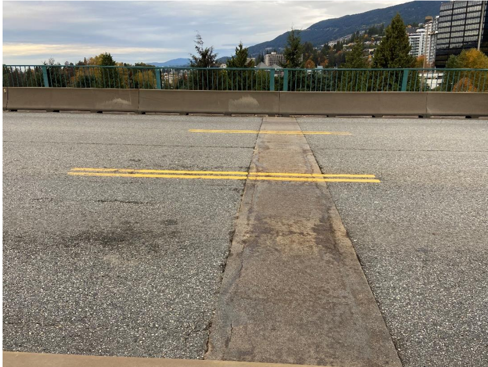
Figure 6: Typical Cracking in Wearing Surface at Link Plates.
