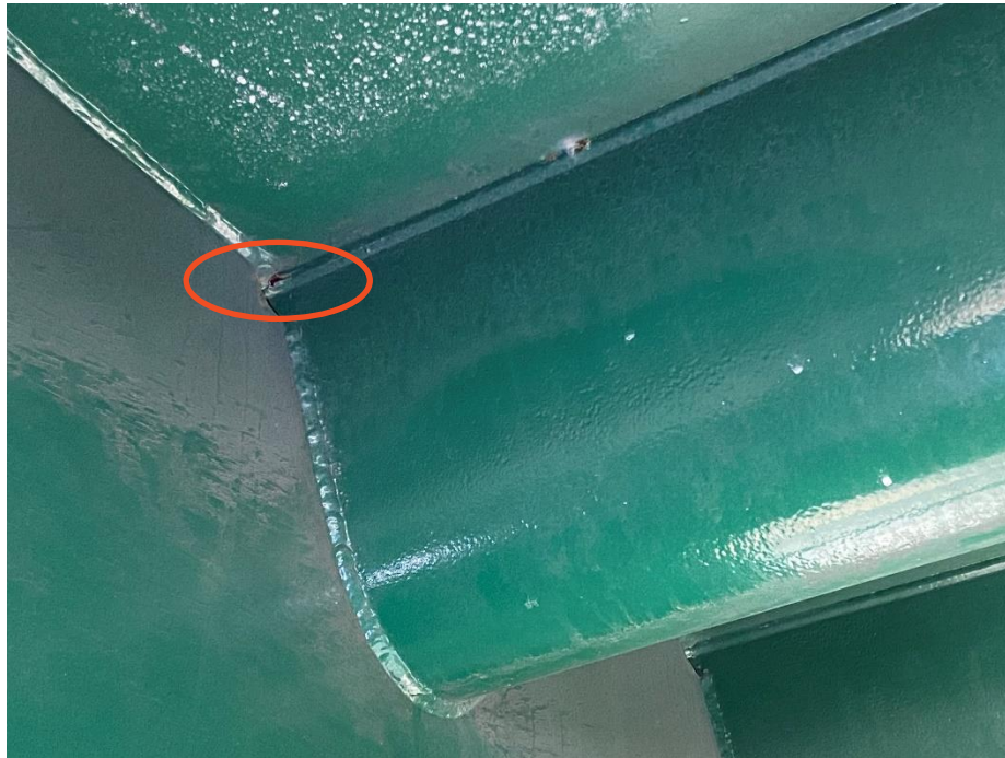
Figure 10: Localized Paint Failure at Termination of Longitudinal Weld on West Side of Trough 6 at 3rd Floorbeam from Bent 4 in the Direction of Bent 5.
