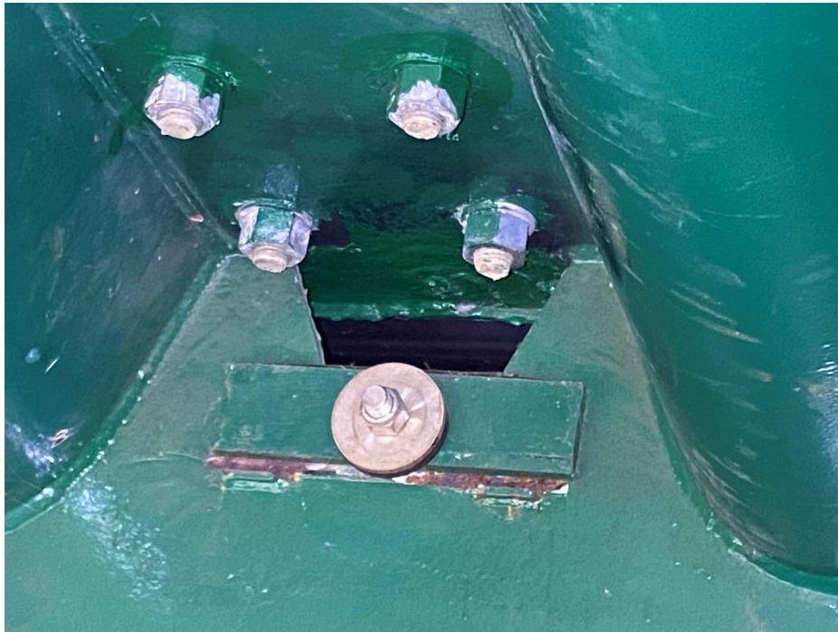
Figure 21: Evidence of Movement of Drainage Trough at Expansion Joint at Bent 9.
