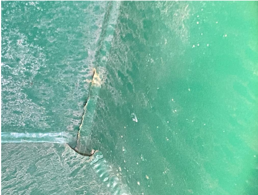
Figure 12: Paint Deterioration at Termination of Longitudinal Weld on West Side of Trough 4 at 4th Floorbeam from Bent 10 in Direction of Bent 9.
