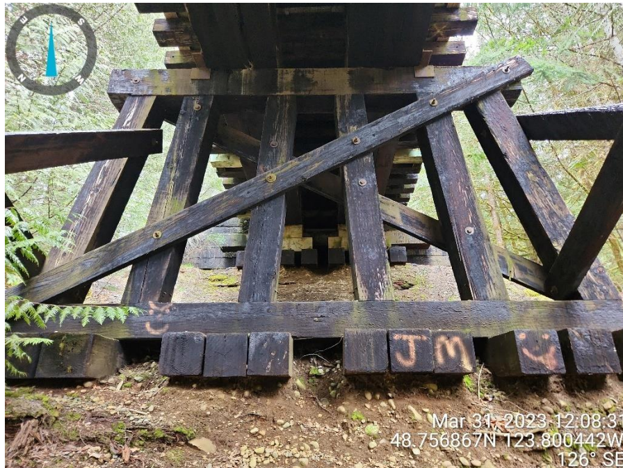
Photo 2 Existing creosote timbers and concrete footings located within the riparian habitat, Facing southeast.
