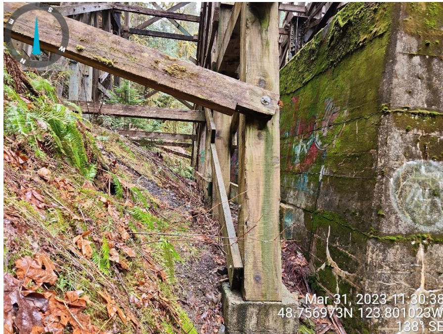
Photo 7 Bridge components (small concrete footings and timber supports) are to be removed. Facing southeast.
