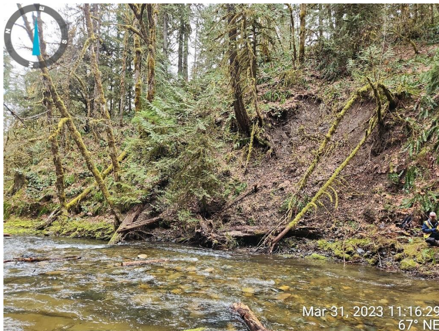
Photo 12 Erosion of the east bank located downstream from the bridge. Facing northeast.
