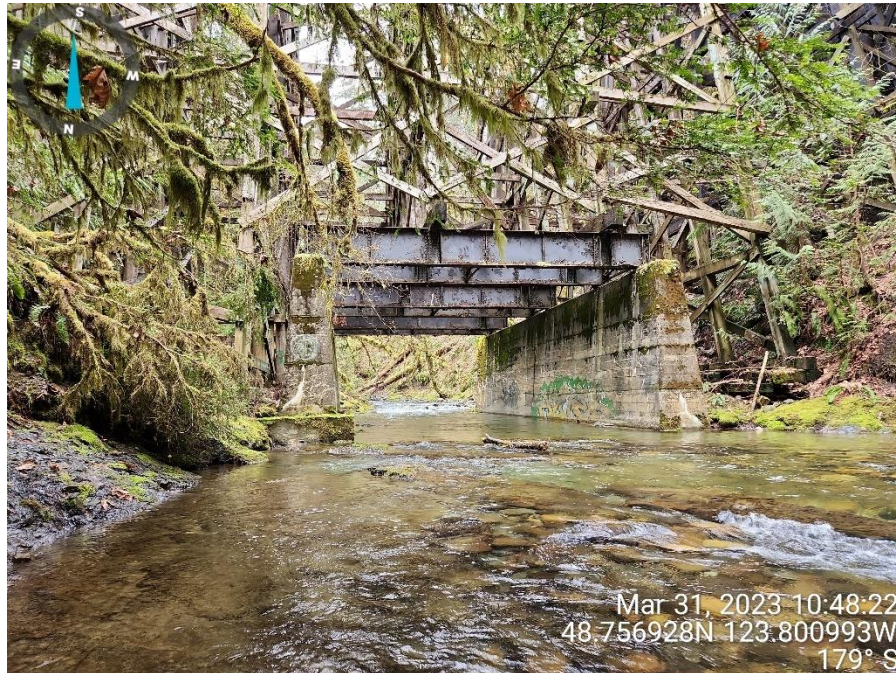
Photo 4 Existing instream footings (to remain) supporting steel beams and wooden trestle. Facing southwest.
