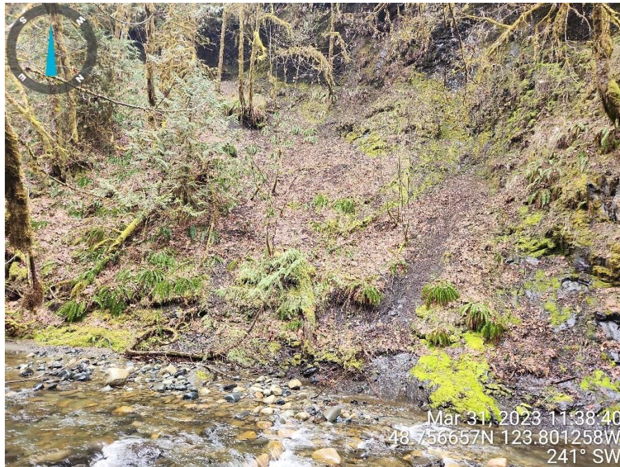
Photo 11 Erosion of the west bank observed upstream from the bridge. Facing southwest.
