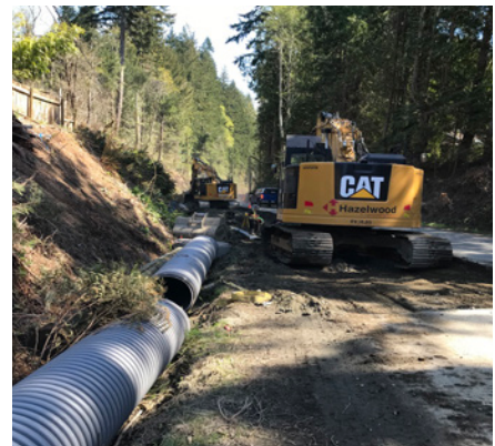
Image 12: Drainage upgrades on Hwy 14 to make our transportation network more resilient to climate change
