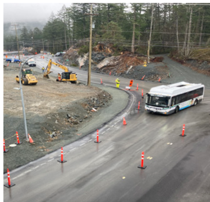
Image 5: Connie to Glinz Lake/Hwy 14 Project, with Park & Ride, and pedestrian underpass. Substantial completion December 2022.
