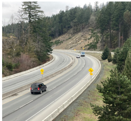
Image 8: Construction of the Leigh Road/Hwy 1 four-laning and median barrier. Completed in late 2020 in Sooke.
