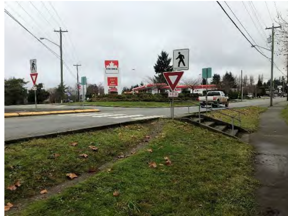
Beaver Creek Road Steps from Sidewalk to Roadway are inaccessible
