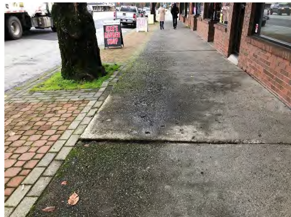
Uneven Sidewalk is a Trip Hazard
