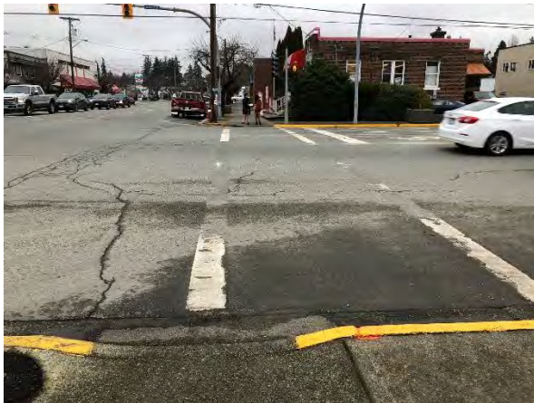
Misalignment of Curb Ramp and Crosswalk Lines
