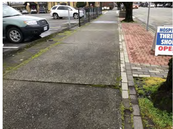
Root Structure Disrupting the Sidewalk
