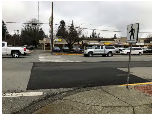
Recent Repaving Missing Pavement Markings
