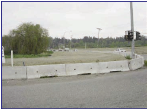
At the 88th Avenue Intersection, preload for the future right turn lane has been placed to the current property limits.
