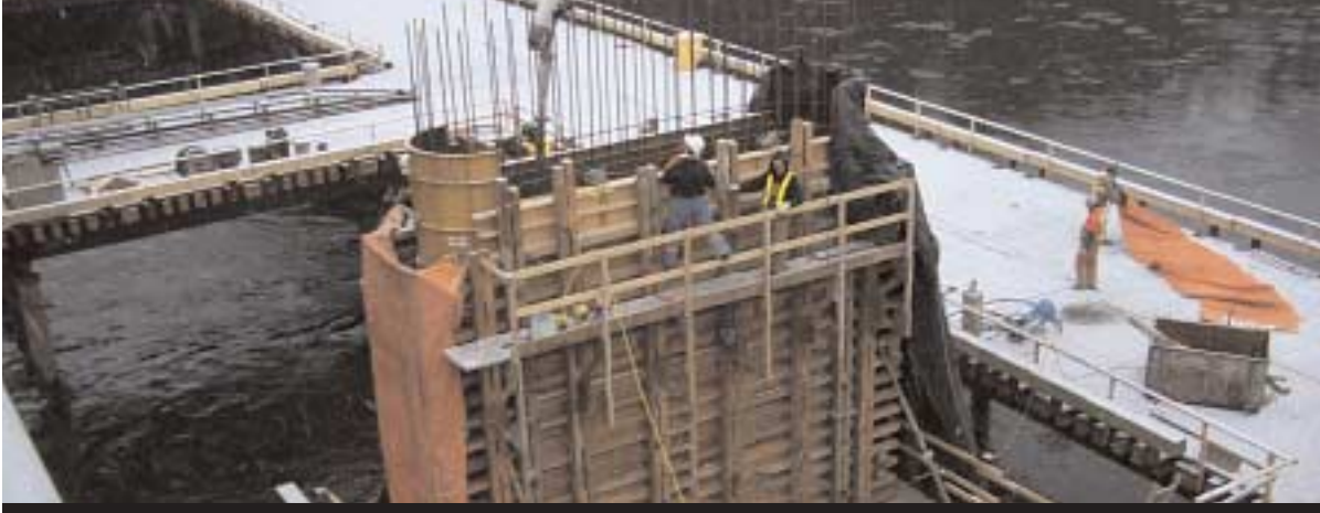
Pouring concrete into a pier form on the new John Hart Bridge
