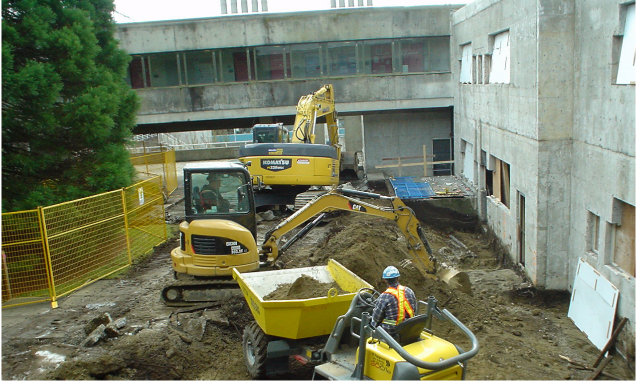
A $49.4-million KIP renovation of Burnaby's chemistry building in the Shrum Science Centre, built in 1965, is creating state-of-the-art facilities and generating 316 jobs.
