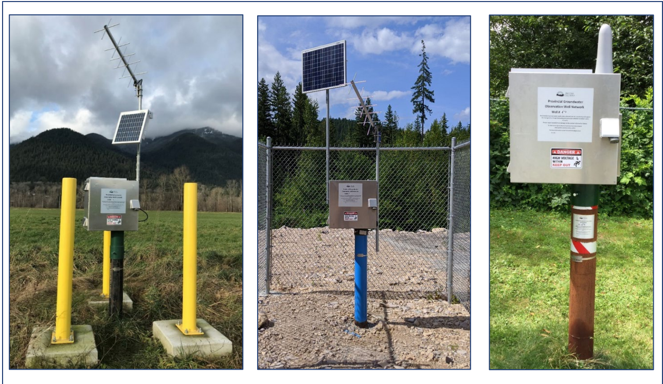
Figure 2-6 Examples of PGOWN telemetry stations.
