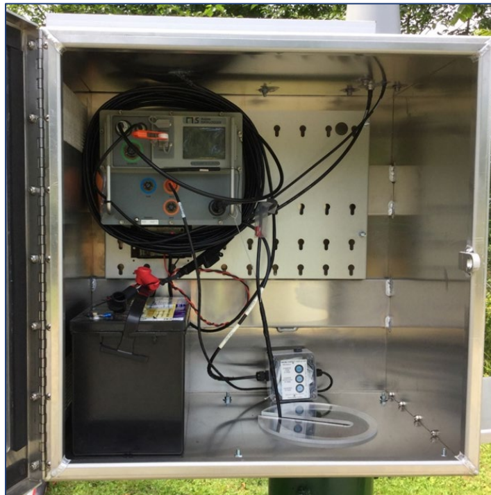
Figure 2-7 Inside a typical telemetry station wellhead cabinet (datalogger, desiccant enclosure, vented direct-read cable, and battery are visible).
