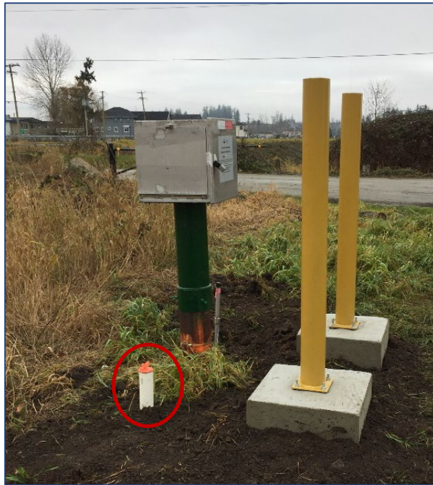
Figure 2-4 Example of a barometric well next to a Provincial Observation Well.
