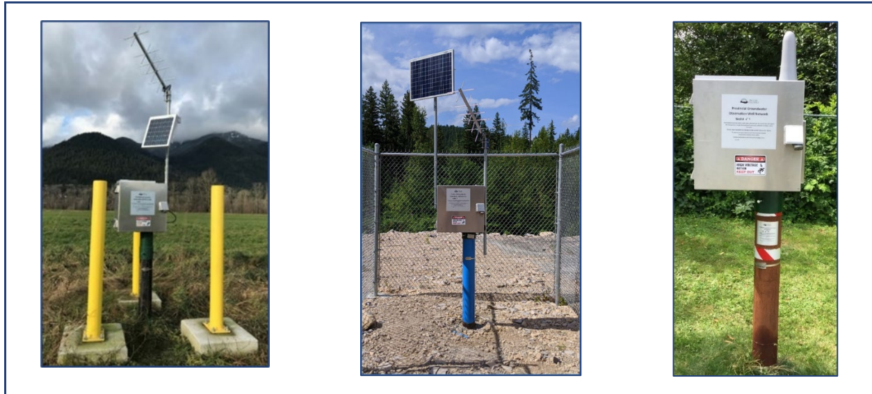
Figure A2-2.1 Examples of telemetry stations.
