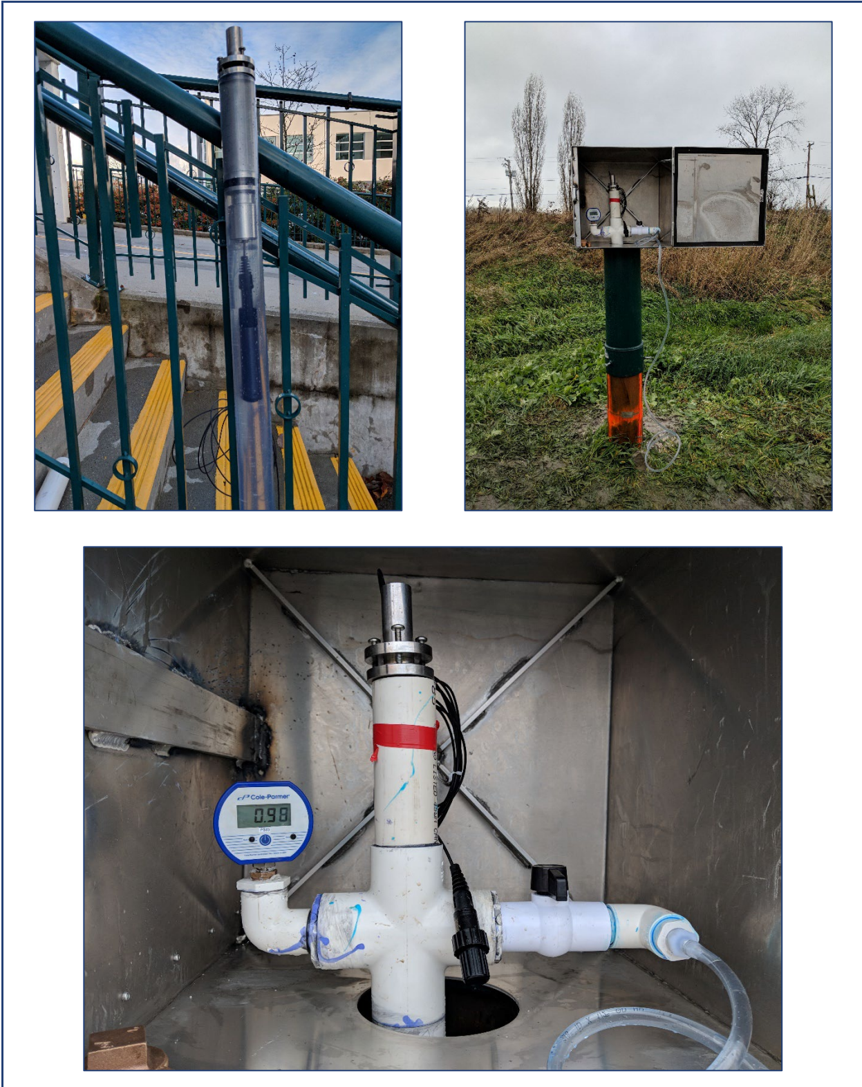
Figure 5-3 Example of an artesian Provincial Observation wellhead.
