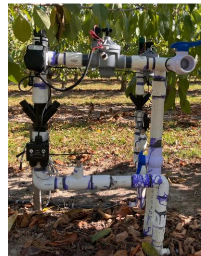
Figure 1. Irrigation valve, retrofitted with Verdi zone level irrigation controller.
