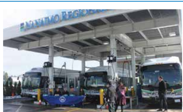
A CNG fuelling station with CNG buses in Nanaimo (photo courtesy Regional District of Nanaimo)
