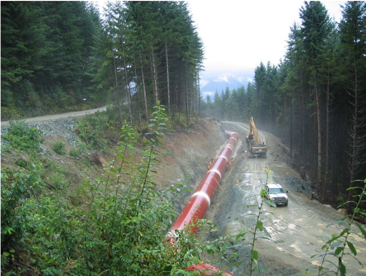
Upper Mamquam Waterpower Project, Squamish Forest District Penstock Installation Below Mamquam Forest Service Road, September 2004
