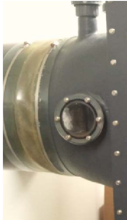
Figure 1: An accumulation of unknown crystals can be seen through the window of this perchloric acid fume hood scrubber system. Deposits such as this must be avoided and carefully removed.
