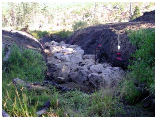
Figure 8. The Esperon Road site showing first lift of large riprap before topping with crushed aggregate. Arrow indicates design height of fill.
