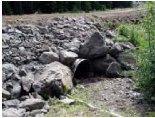
Figure 12. Inlet of arch showing placement of large and small riprap on fill slopes around the arch.
