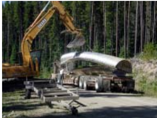
Figure 4. Lifting arch off delivery truck in preparation for placement on small trailer.
