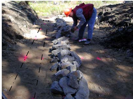
Figure 10. Windrowed riprap along culvert centreline. The white dashed lines show where paint lines would indicate the location for one side of the arch's footings.
