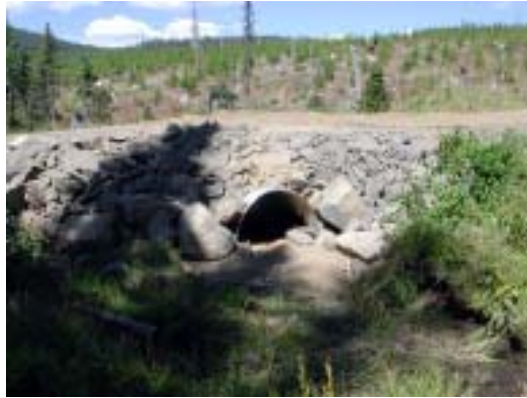
Figure 13. Outlet of arch at Esperon Road site showing fill height above arch and the low areas on either side of the arch along the road.
