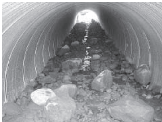
Figure 9. Simulated streambed within CSP, showing range of material sizes and a low-flow channel.
