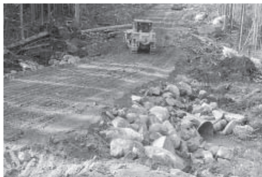
Figure 8. Riprap armouring at outlet and final road grade showing fill height over the embedded CSP.
