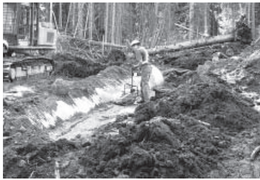
Figure 6. A plate compactor was used to compact backfill lifts on either side of the CSP.
