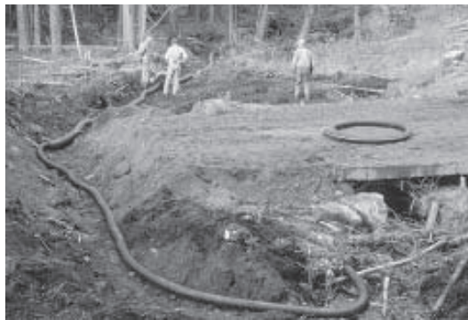
Figure 2. Diversion pipe laid in a trench on the bush side of the temporary structure.
