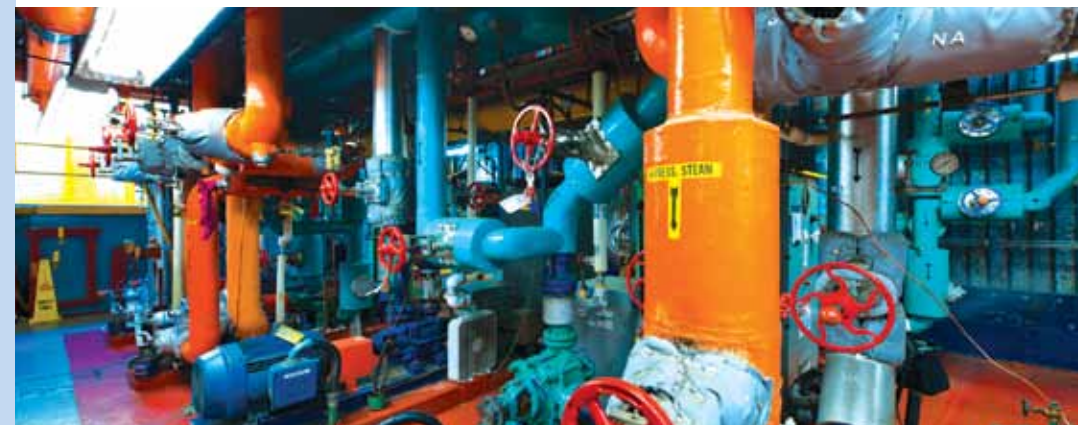
University of British Columbia, District hot water system
