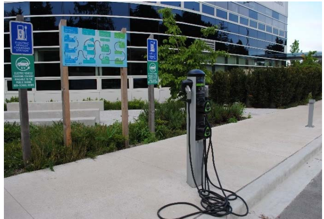
With partner grant funding, electric vehicle charging stations were installed at two schools.
