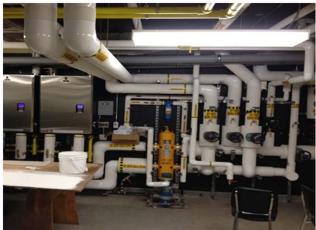
A modern heating plant at Fraser Elementary has improved comfort and will reduce energy costs and greenhouse gas emissions.
