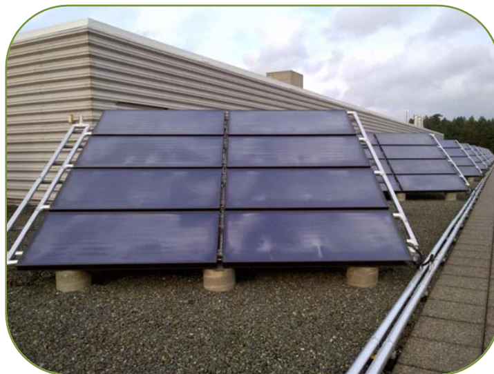
Solar Collectors at Victoria General –Operating since Dec 1, 2011
