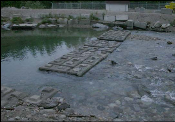
Plate 2. A cross-section view of the weir in Swift Creek. This weir has helped to increase water storage capacity in Swift Creek.
