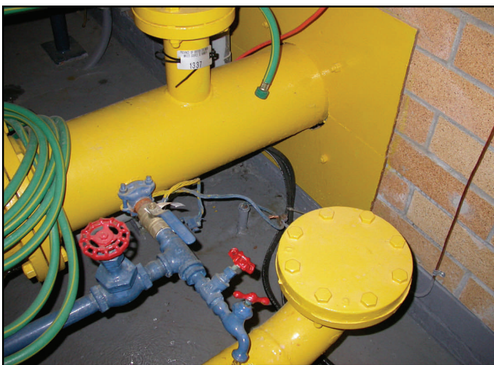
Plate 2. A picture of the raw water tap inside the Mackenzie pump house.
