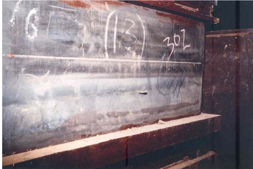
Figure C11.6.6.8.f.3 Loss of bonding between two layers of rubber. Note the coin inserted into a crack
