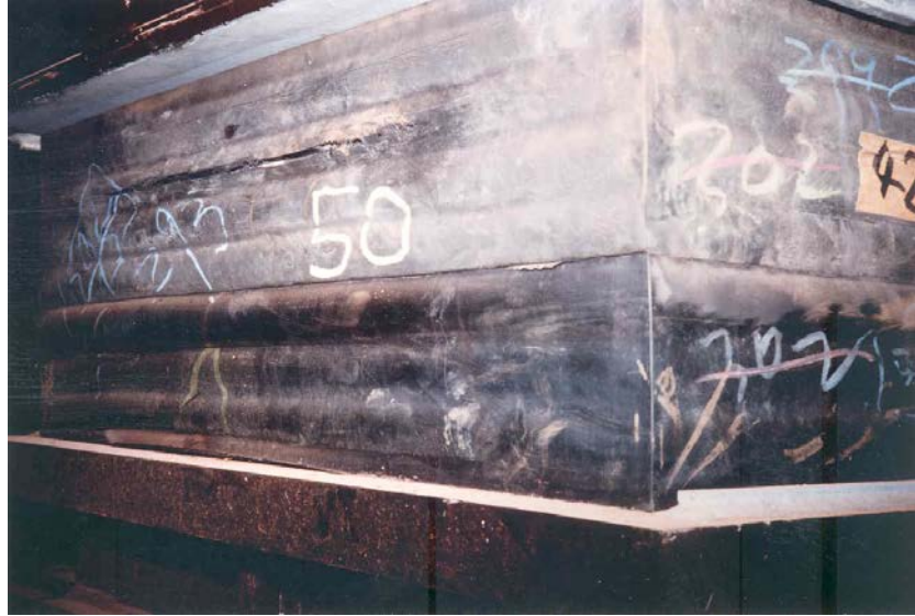
Figure C11.6.6.8.f.1 Splitting along a bulge (above the number 50)
