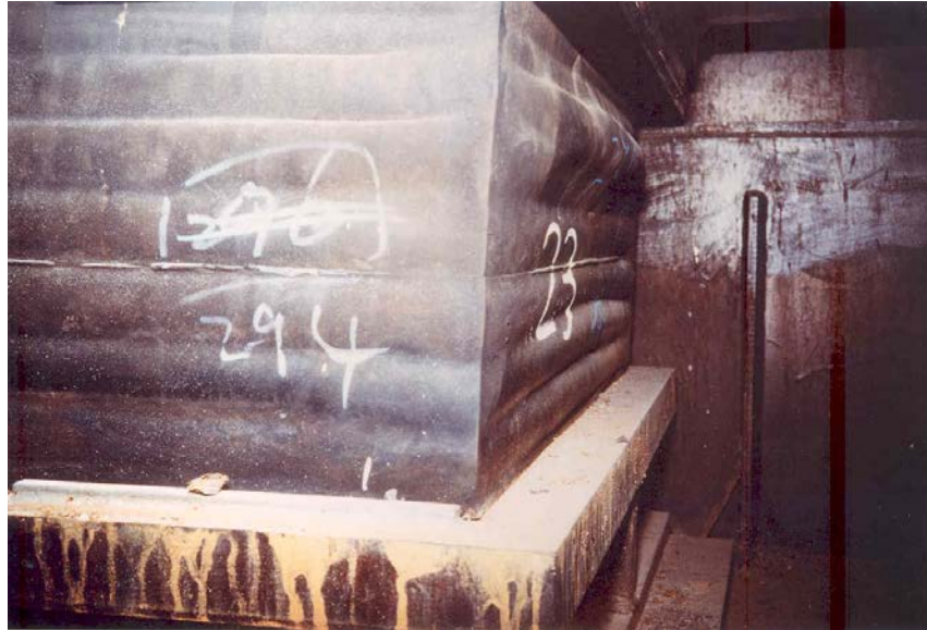
Figure C11.6.6.8.f.5 Loss of bond between two rubber layers
