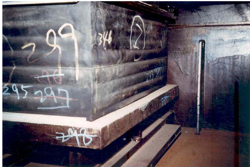
Figure C11.6.6.8.f.2 “Roll out” of the bottom of the bearing along the right face, possibly because the thickness of the lowest layer of rubber was too thick
