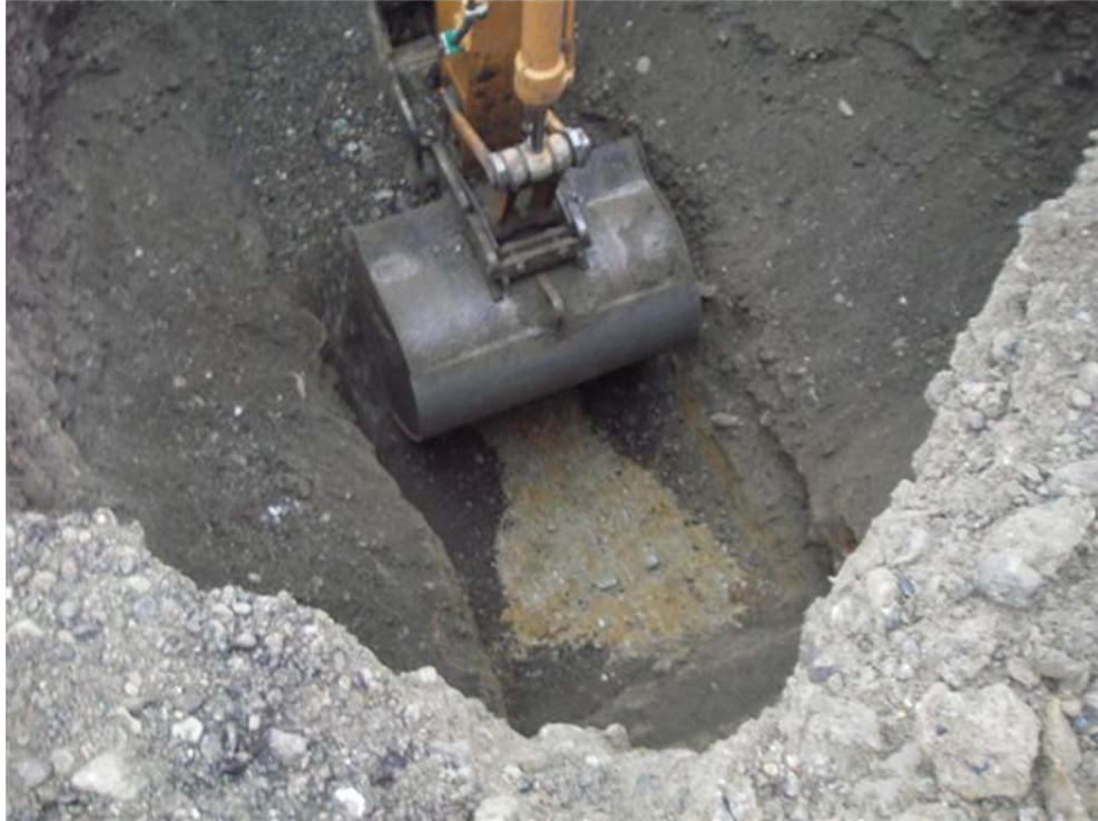
Underlying poor quality material at depth.
