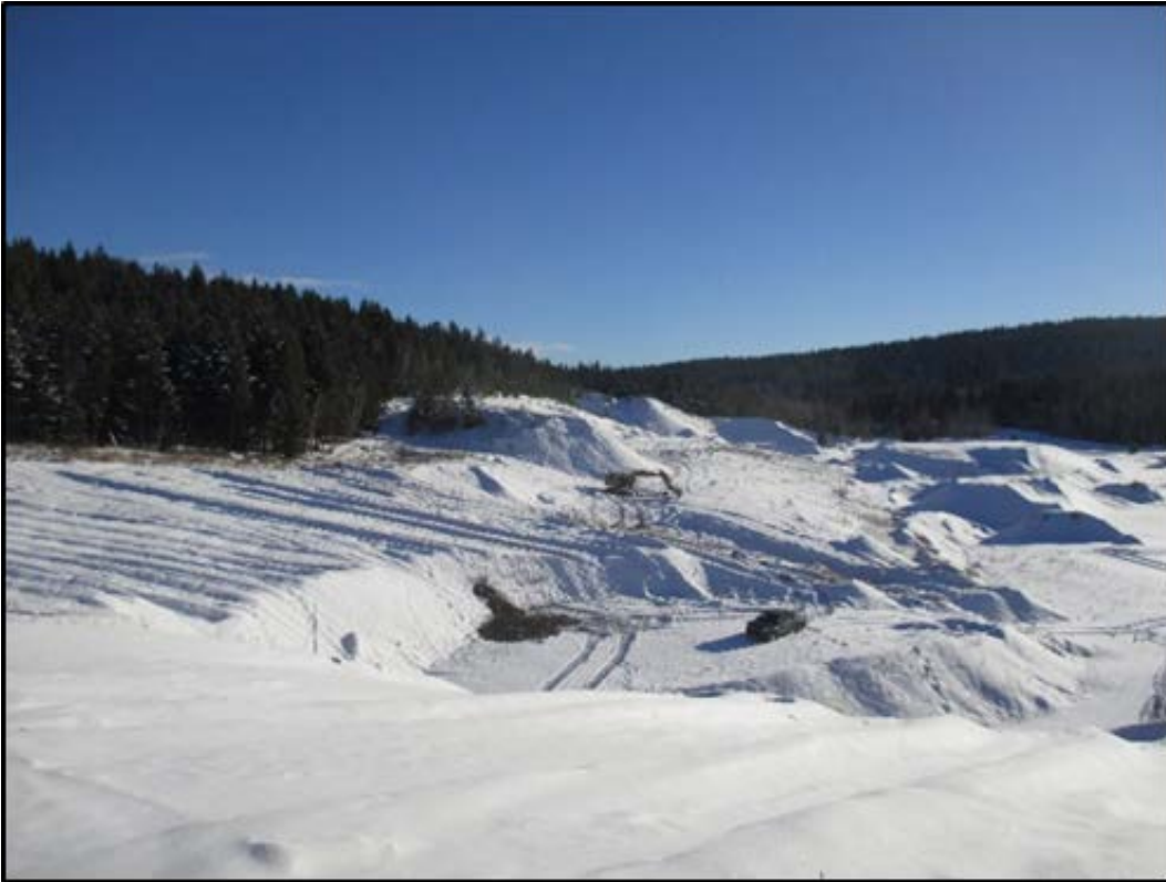
Crusher location at base of slope to right of pickup, mining area to left and foreground, with aggregate stockpile area on right.
